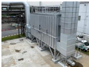
RTO Regenerative Thermal Oxidizer
